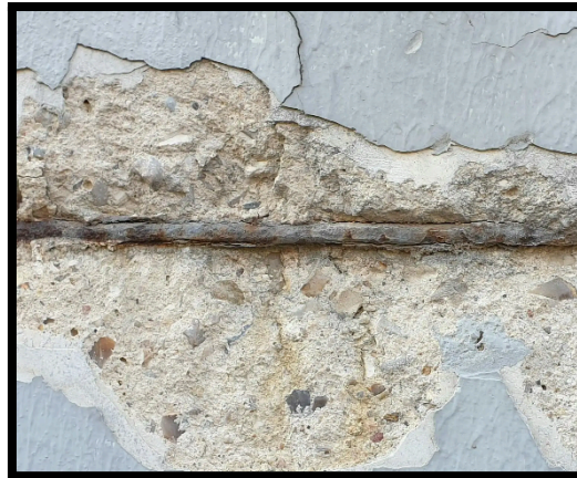
Gambar 6. Concrete collapses due to the pressure exerted by oxides on the surface of the reinforcing steel, which enlarge and thicken over time. (Web-6)
